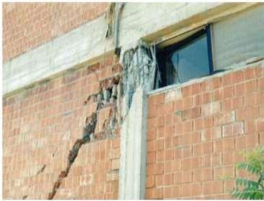
Figure 1.5: Short column failure [2]
