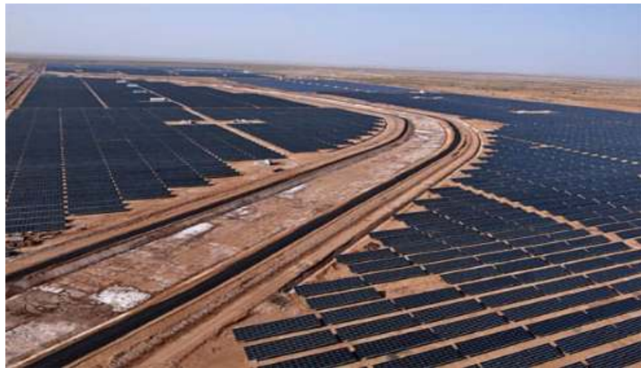
Figure 12(charanka solar plant)
